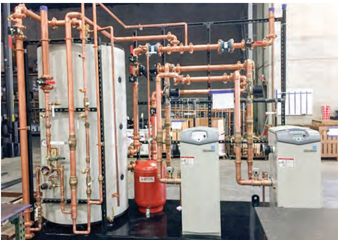
With the ManufactOn cloud and mobile solution, TG Gallagher has increased and improved its prefabrication capacity. This finished assembly was managed and tracked through ManufactOn.
