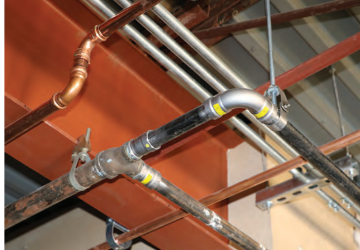
Braconier ran nearly 5,000' of new piping in the renovation and expansion of the Aims Community College welding building. It was estimated that pressing with Viega cut at least a week off the installation time in the welding lab alone.
