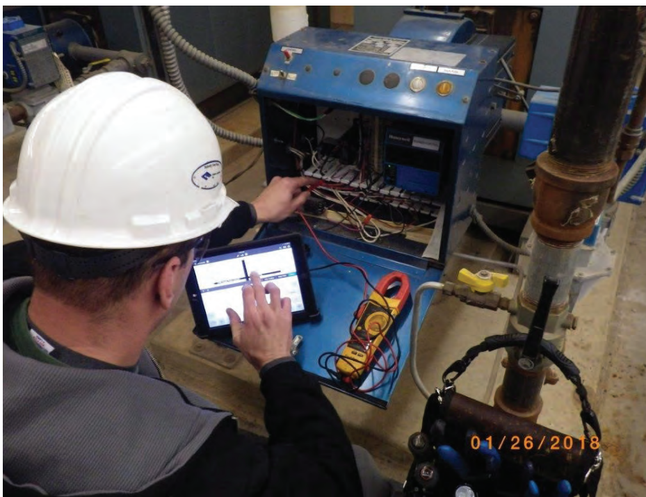
Goshen Mechanical Technician Ben Shumoski enters system data in MobiliForms for immediate processing by Goshen’s main office. By using MobiliForms, Goshen has eliminated lost work orders and sped up payments.
