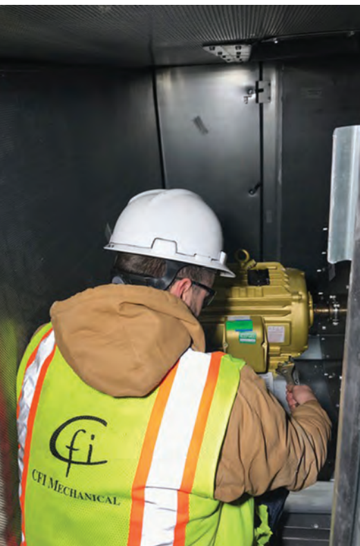
A CFI Mechanical technician installs a motor for a new air handling unit for Northside High School, one of several Carrier products selected to provide high-efficiency, low-maintenance cooling in warm, humid Houston—and to help the school qualify for LEED status.
