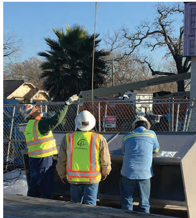
With a total timeline of 18 months for the Northside High School renovation, often while school is in session, CFI Mechanical is working closely with Carrier on a just-in-time delivery schedule, so HVAC components are sent to the project's lay-down areas at prescribed times, saving the contractor both time and related installation costs.
