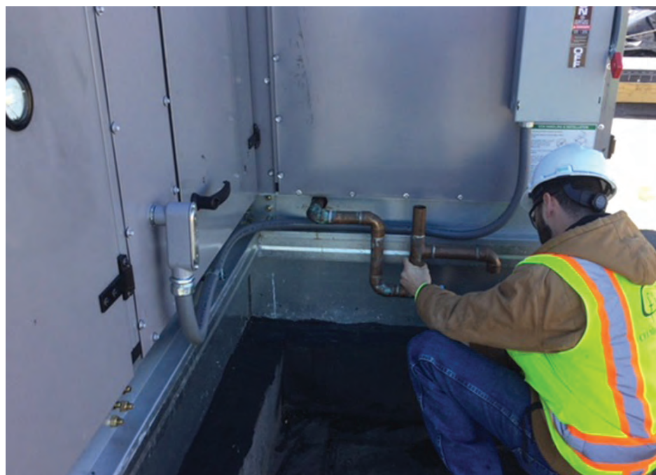
CFI Mechanical chose Carrier equipment, such as the air handling unit shown here, to provide Houston's Northside High School with reliable and precise comfort for its students, faculty, and staff, with a minimum of time and effort invested by the school's maintenance staff.
