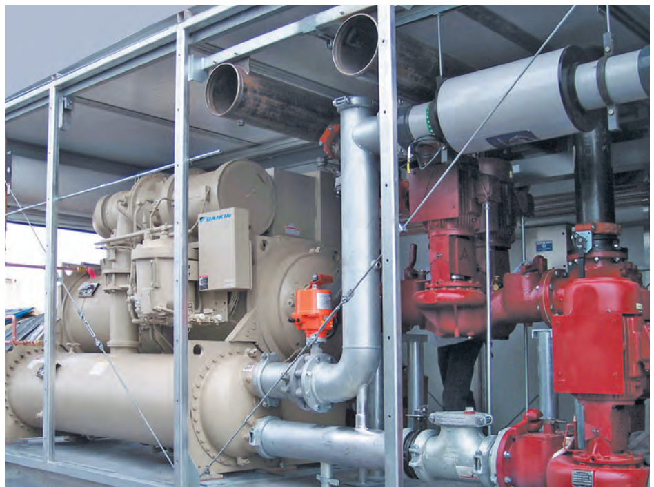
Each of the Daikin Modular Central Plants consists of a 500-ton Daikin centrifugal chiller pre-engineered with pumps, piping, cooling tower, control panel and associated water treatment system. Because they were pre-assembled, these four modules were successfully installed in just one week, resulting in no downtime for Herakles Data.
