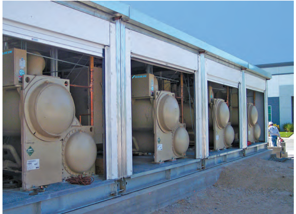
Installing Daikin Modular Central Plants not only met Herakles Data’s high-capacity cooling demands but also cut their energy use, earning the company a $50,000 municipal rebate.
