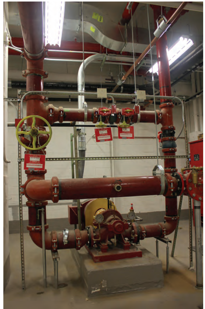
Combining Victaulic's grooved mechanical couplings with its CPS solutions significantly sped up Martin Associates' installation of an HVAC system for a new luxury apartment building in New York City. The Victaulic CPS team and Martin Associates worked closely together to fine-tune the building's piping system designs, utilizing every available inch of the tight mechanical space.
