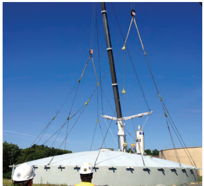
Wire rope slings are complex machines that should be inspected and maintained to ensure safe use.
