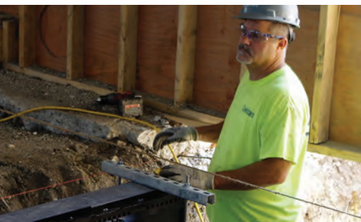
A worker begins installation of a Smith Enviro-Flo® II Trench Drain System in the facility that will be Cannistraro's manufacturing facility for plumbing, HVAC piping, fire protection, and sheet metal trades. Cannistraro was so impressed by Smith products and services that they named Smith their supplier of choice.
